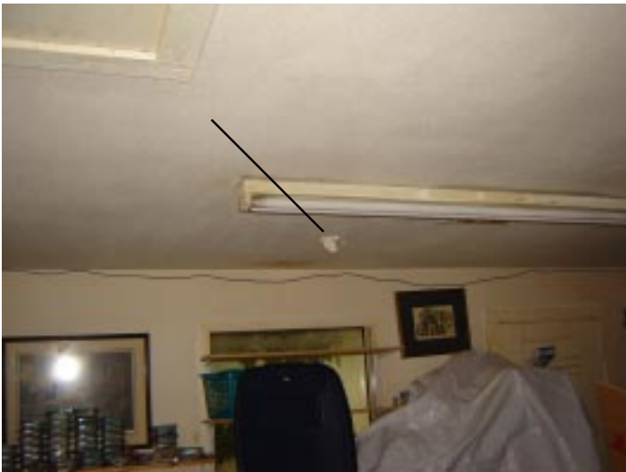
A branch came through the roof of my home office and a little punched through the ceiling. A lot of water came through that little hole.
