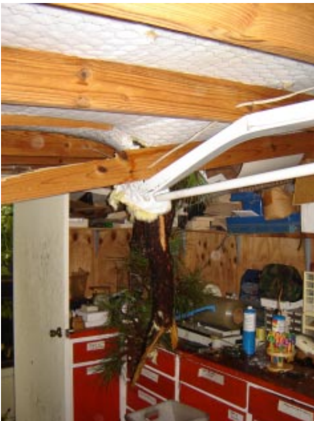
8" limb that came through shop/storage area
