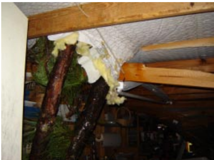
A large branch came through the front part of the shop/storage area.
