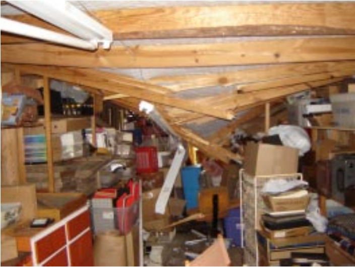
My shop and storage area was in shambles. The structure is totally destroyed but most contents were saved.
